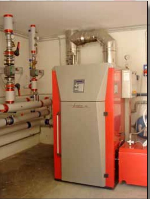
110kw Sommerauer&Lindner wood chip boiler
