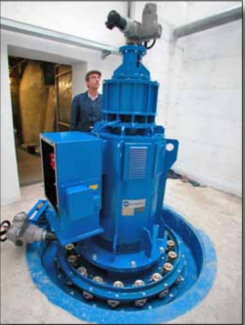
160 kwh Kaplan turbine hydroelectric power plant
